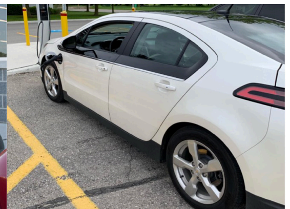
On-site EV charging capability.
